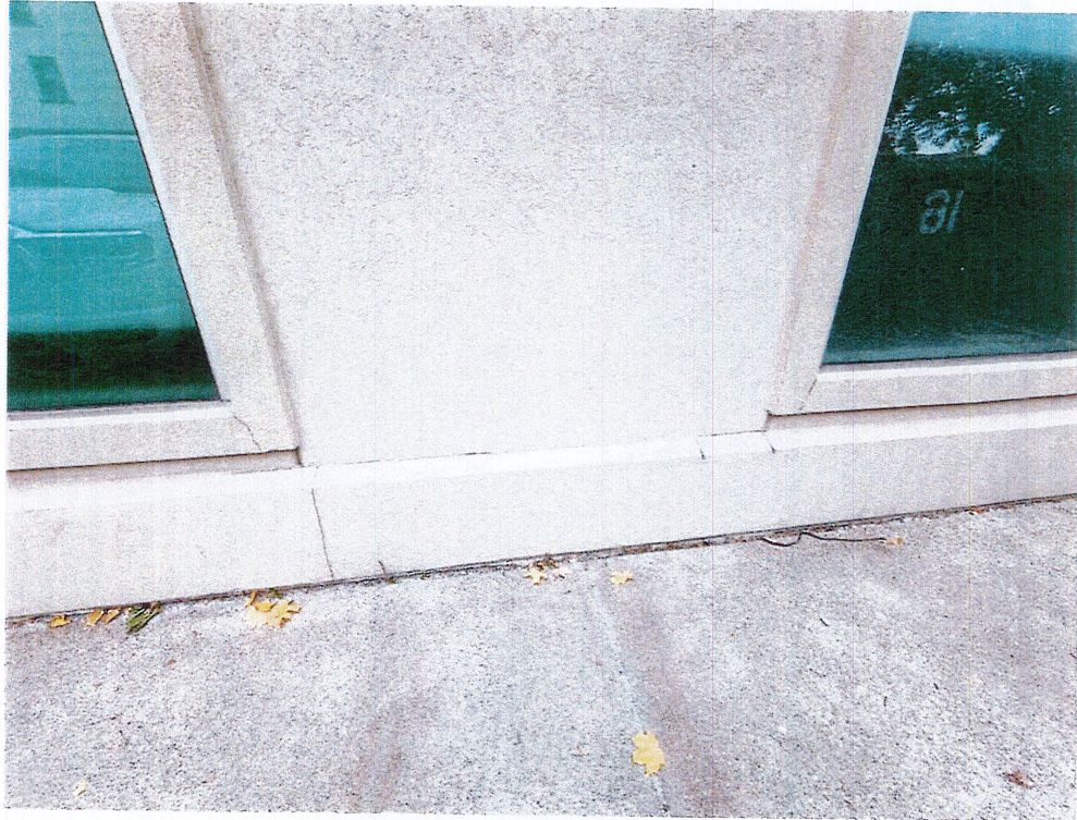
Exterior EIFS cracks at windows
