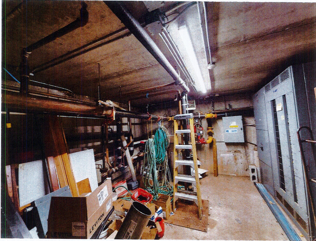
Main electrical room
