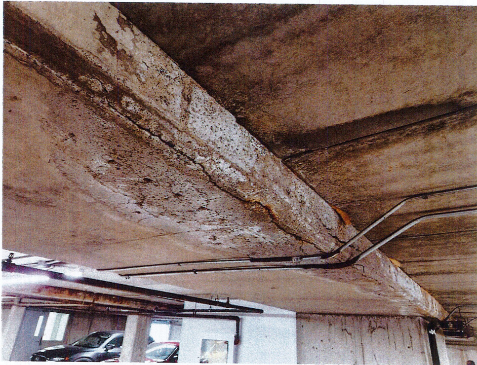
Concrete beam delamination at parking deck
