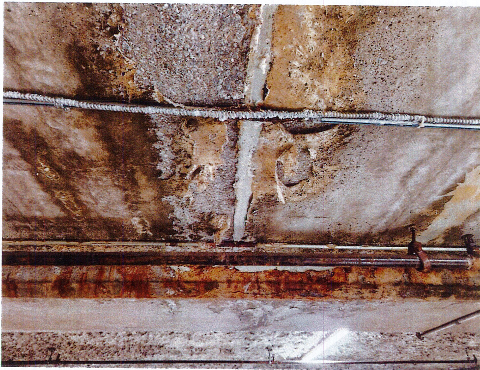
Concrete beam delamination at parking deck
