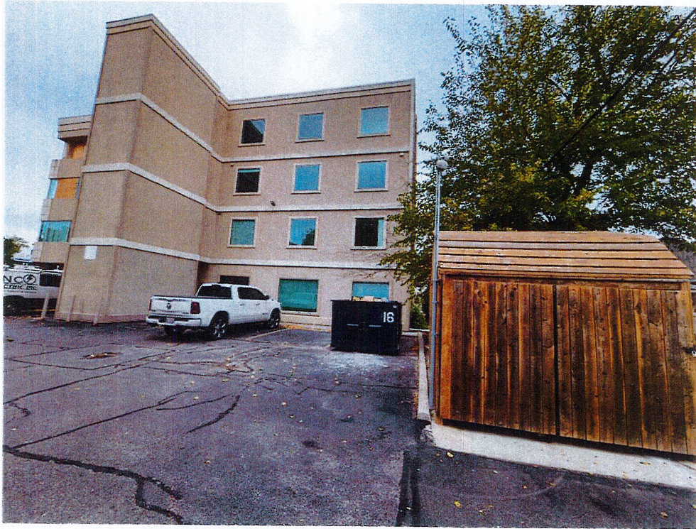
Exterior EIFS façade (deteriorated asphalt pavement)
