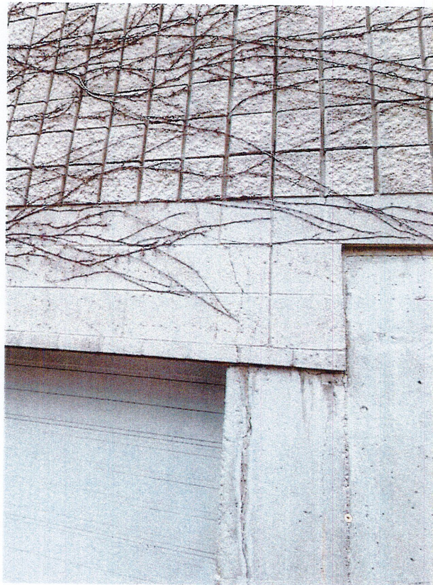
Exterior block cracks at overhead door
